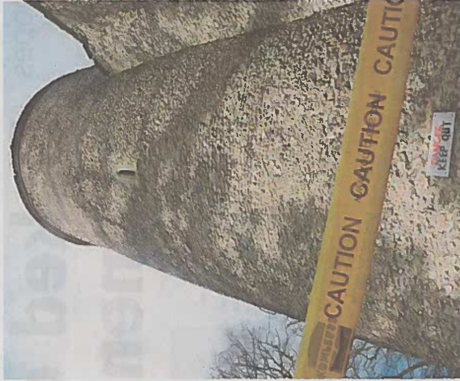
AT RISK: The faulty church tower.
